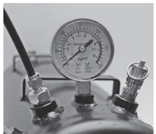
Fig. 5 High-pressure plastic hose connected
