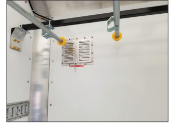
Front Wall Vents
