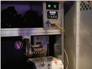
Auxiliary Power Systems
