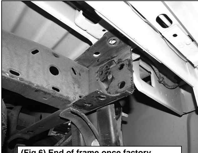
(Fig 6) End of frame once factory bumper is removed. Passenger side w/o receiver hitch pictured
