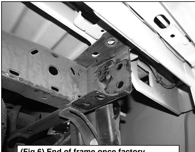
(Fig 6) End of frame once factory bumper is removed. Passenger side w-o receiver hitch pictured
