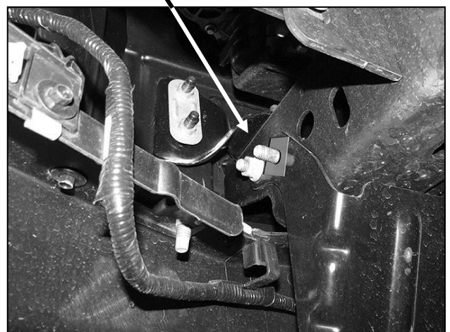
(Fig 9) Driver/left frame extension pictured
