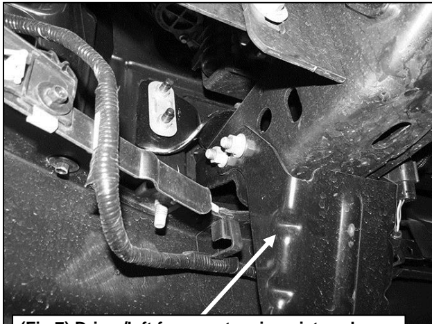
(Fig 7) Driver/left frame extension pictured
