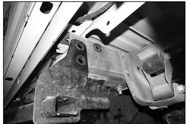
(Fig 7) End of frame once factory bumper is removed. Passenger side with receiver hitch pictured
