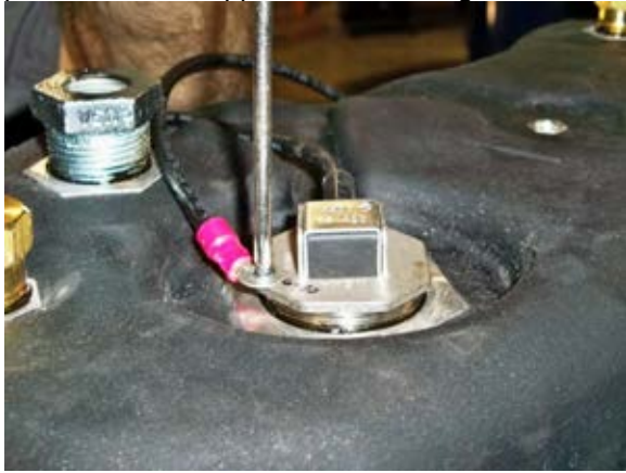
(Fig. 8) Connecting small eyelet end of grounding wire to top of electric fuel sensor. Other end to chassis frame.
