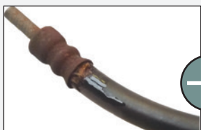
COMMON PROBLEM: Leaking hose at collar
