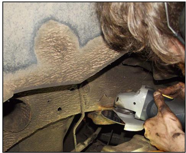
Remove factory bumpstop bracket by grinding the weld off or by using a heavy hammer and chisel to remove the tack weld.
