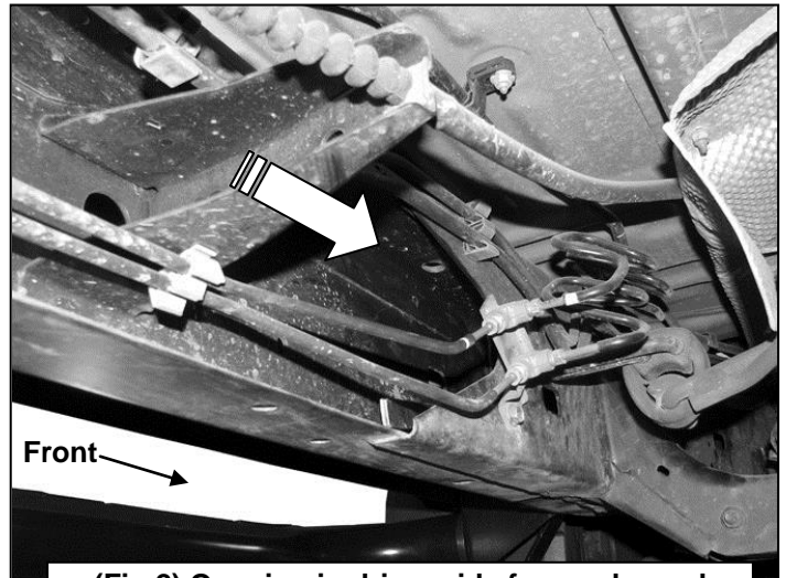
(Fig 2) Opening in driver side frame channel pictured from below and behind frame channel
