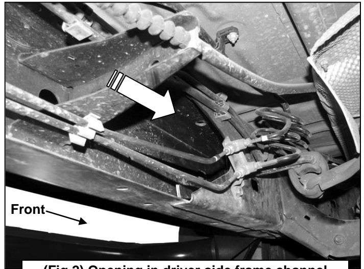
(Fig 2) Opening in driver side frame channel pictured from below and behind frame channel
