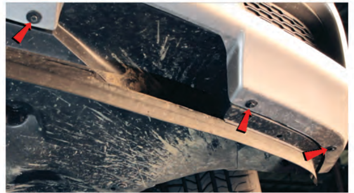
8) Unseat the front bumper fascia by pulling it up to unseat the fascia retainer hooks, then pull the edges out and ease the fascia back.
