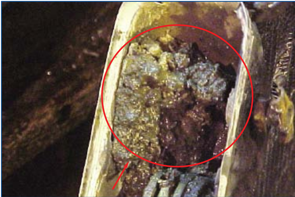
Additives used to stop leakes render warranties null and void
