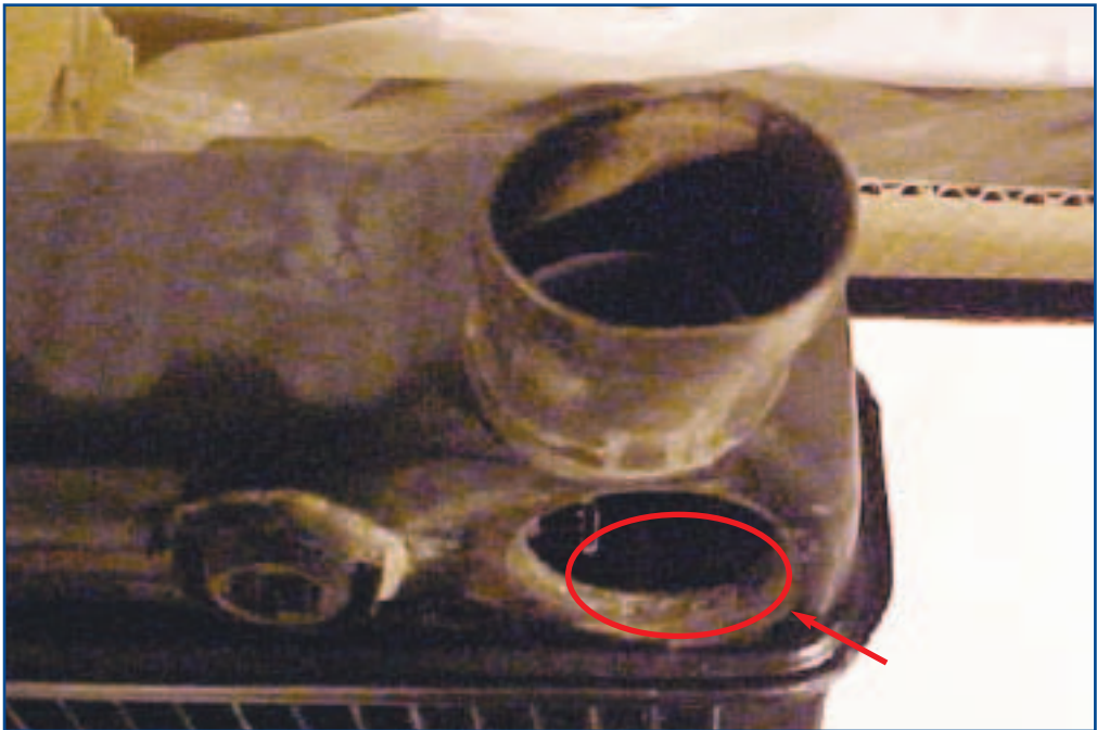
Loose or broken connection due to bad soldering
