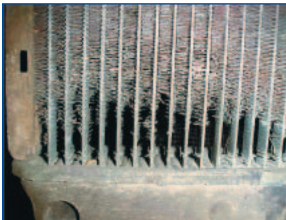
Illustration of Fin Deterioration
