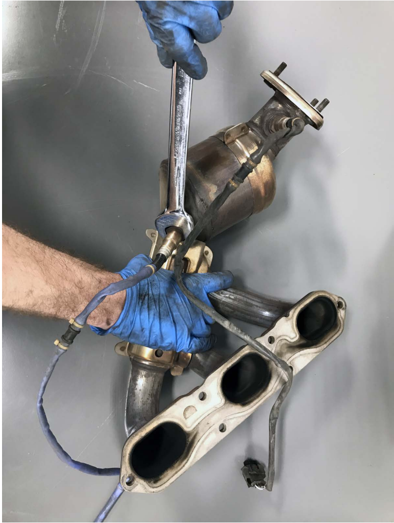
Pictured Above: After removing the factory headers, with them on the ground use a 22mm wrench to remove the oxygen sensors. This may take some time/patience /heat
