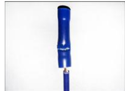
Broken Butt Connectors
