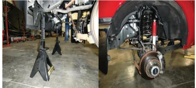
Lift front of vehicle and support with min. 3 ton jack stands. Remove front wheels and tires.
