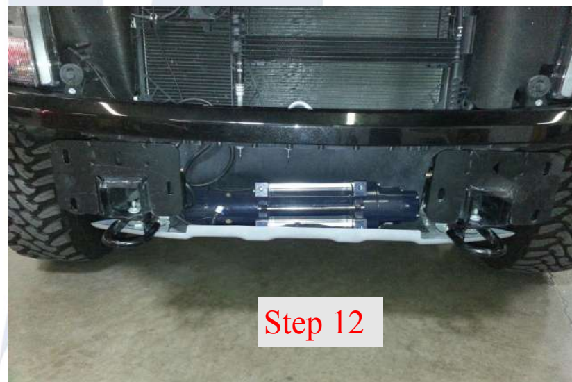
Step 12: Now re install the skid plate to your vehicle. If your going to install a winch the front lip of the skip plate is a good place to hold the winch while you are finishing up the mounting of the bumper.
