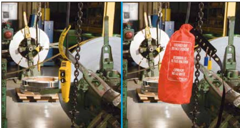
Hoist Control Cover
