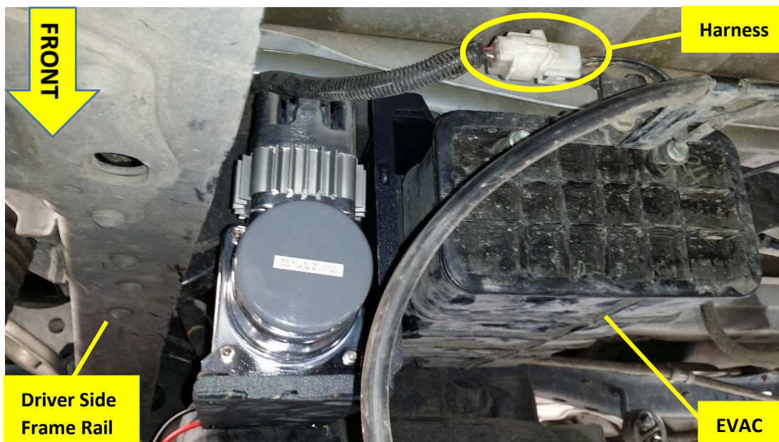
Figure 9 - TUNDRA-301 and Air Compressor Mounted next to EVAC
