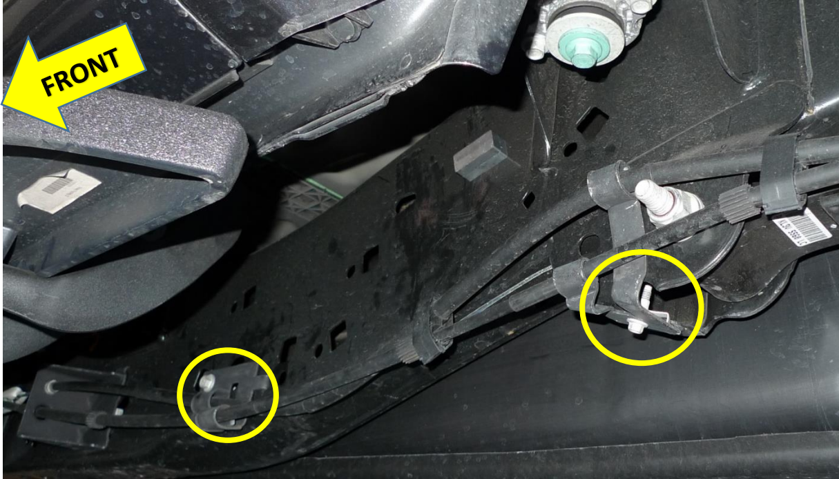
Figure 28 - Driver's Side Frame Rail under rear door
