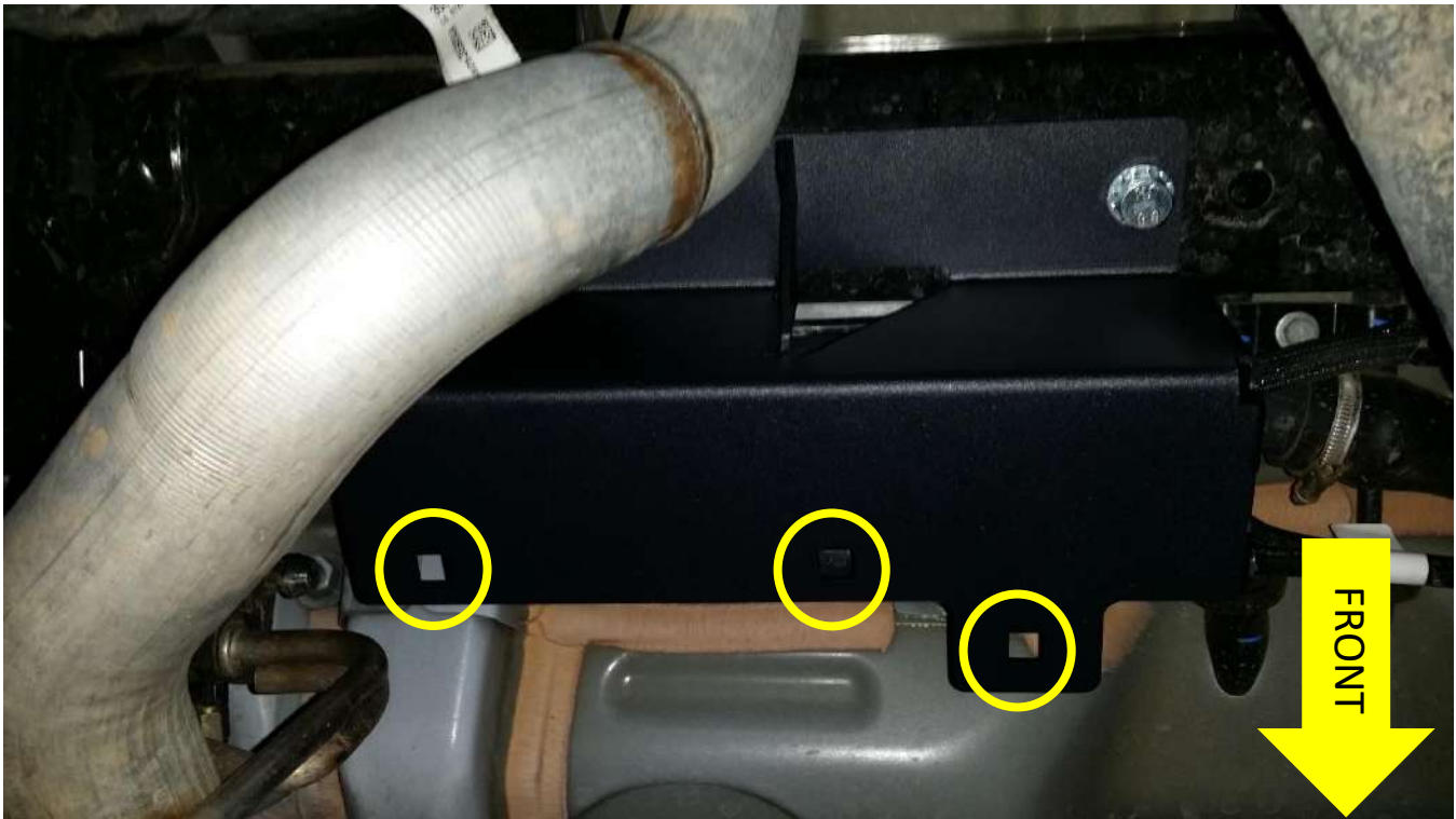
Figure 8 JL-201 Adapter Bracket Bolted in Place
