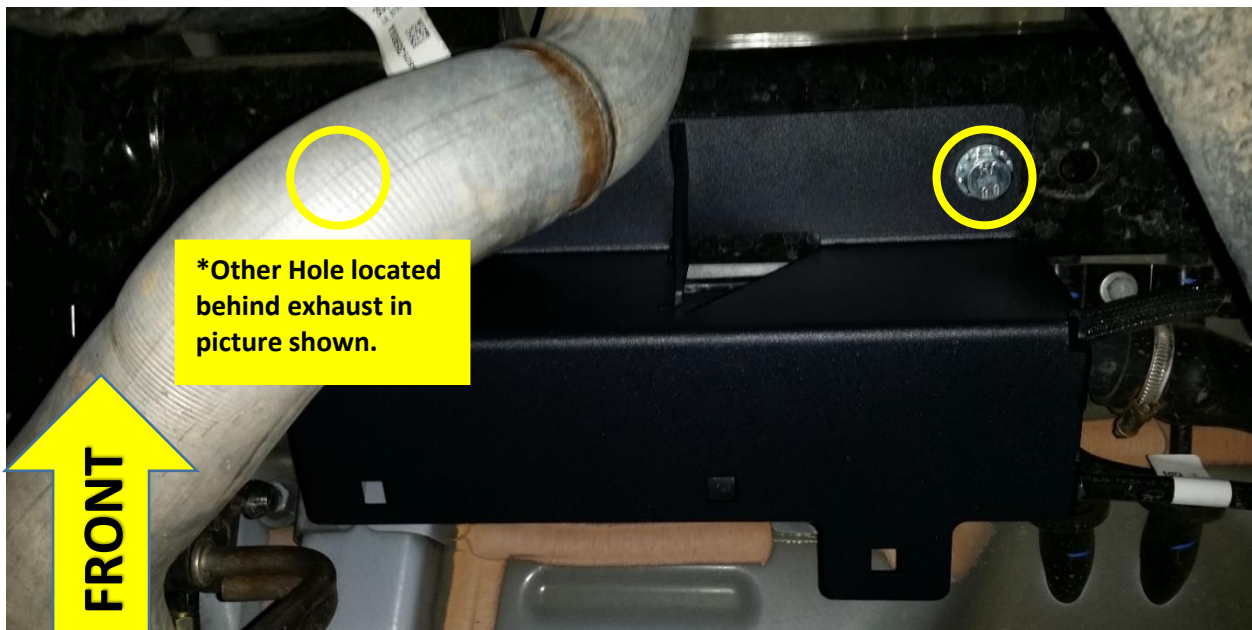
Figure 13 - JL-204 Adapter Bracket Bolted in Place
