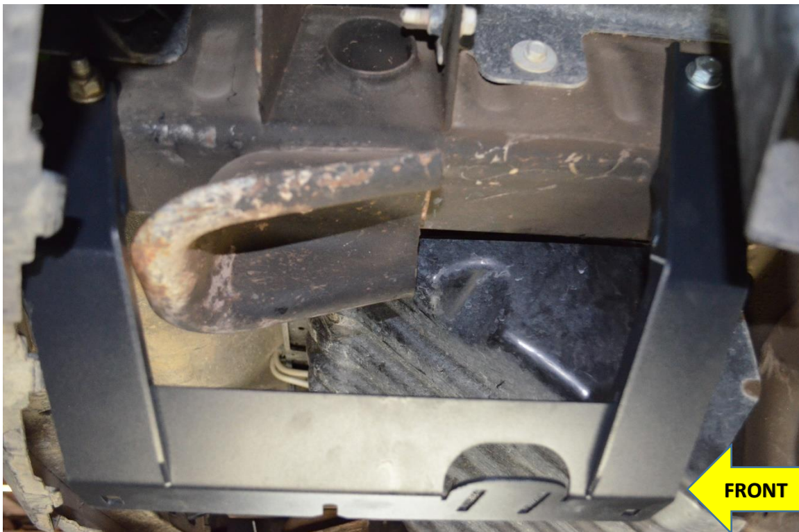
Figure 16 - Bracket Attached to Frame Rail (Driver Side)
