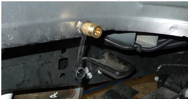
Figure 19 - Compressor to Air Tank Line
