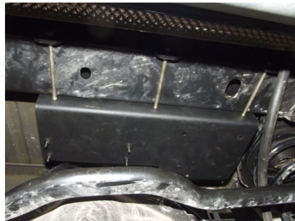
Photo 6 – Mounting bracket, as seen from underneath.
