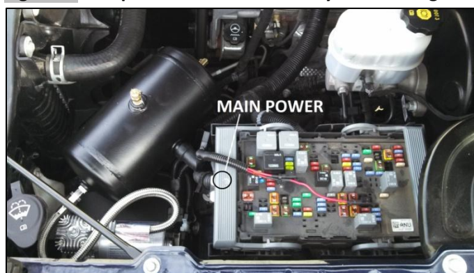
Figure 2: Compressor & Tank Assembly with Wiring:
