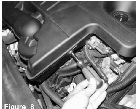
Figure 8 With long 8mm nut driver, loosen the clamp under the engine cover on throttle body.
