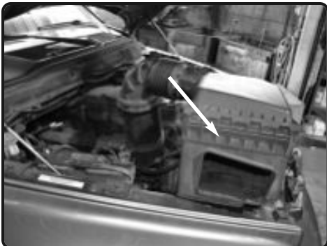
5. Pull the air duct off the turbocharger and then firmly lift up on the entire air box assembly and remove the entire stock air box assembly from the engine bay
