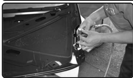
9. Use a flat grinder to straighten the edges and clean up all the metal burrs. Slowly grind back on the open. Only grind what you need for additional clearance. Please use caution and have proper safety equipment like goggles and air respirator!!!
