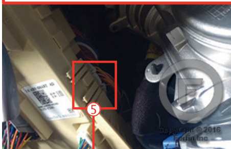
⑤ Back of fuse box
