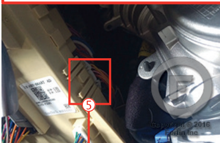
⑤ Back of fuse box
