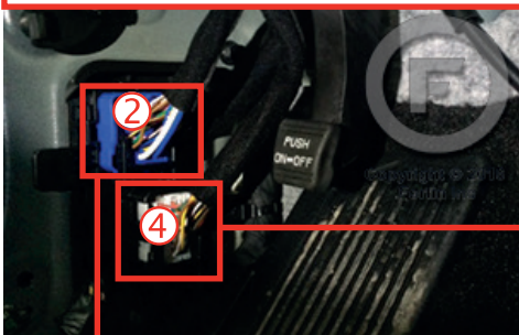
In the driver's side kick panel
