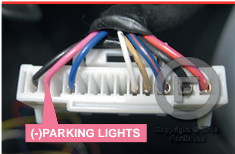
② At parking Lights switch
