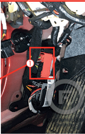
① In the driver's side kick panel
