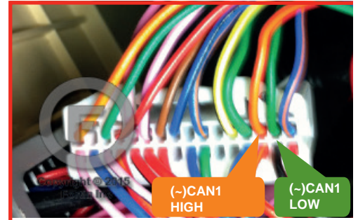
④ Back of fuse box
