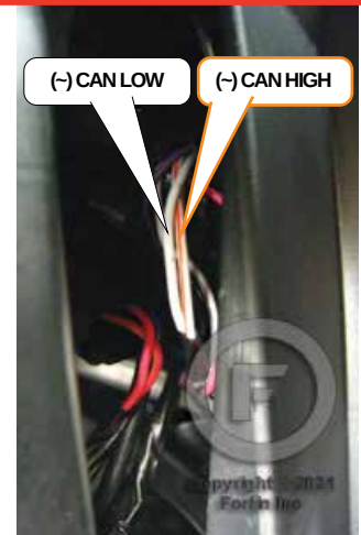
① Back of key switch on dashboard
