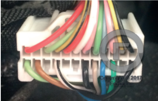
① Under steering column, START-STOP unit.
