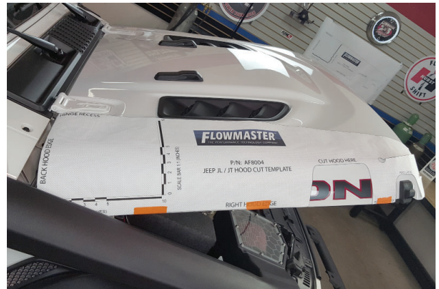
39. Open hood and set template onto it, aligning rear and side edges. Secure bottom edge with tape.
