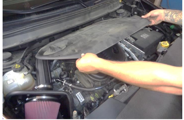
32. Install the engine cover.
