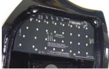
LED board in place.
