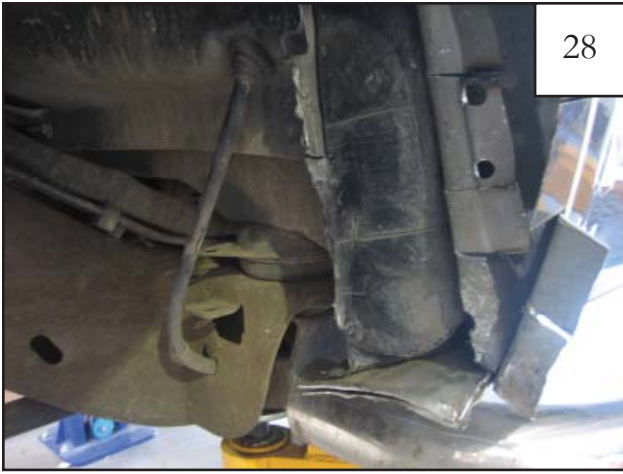
28 Cut pinch seam at mark made in previous step. Bend flange back even with firewall.
