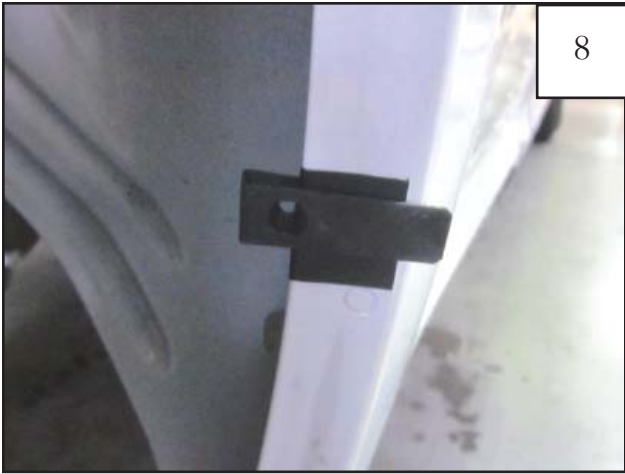
Install a Clip (CL1-0009) over each of the four Tabs (MT1-0034) placed over the upper 4 marks made in Step 16.
