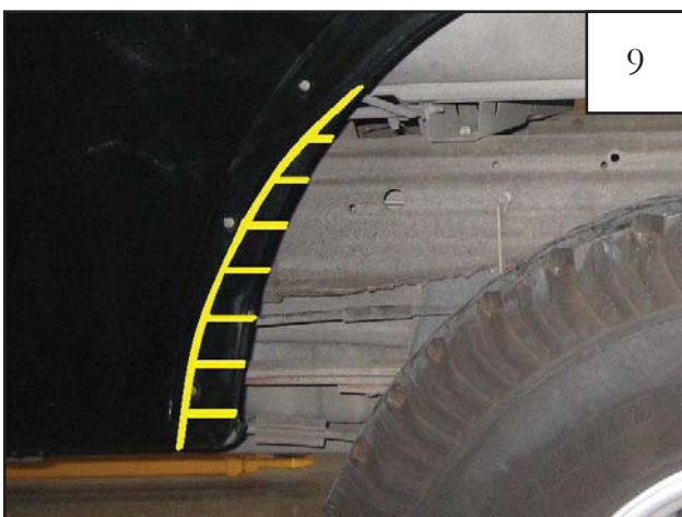
At 1-1/2" intervals, make horizontal lines from fender lip to line drawn in Step 8. These lines will be cut later, forming tabs to be hammered in.
