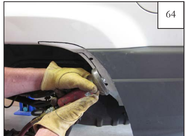
Using a cut off wheel or other suitable tool, cut along line marked in step 63 removing the inner flange.
