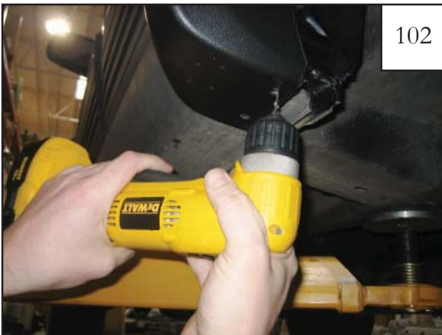
Drill 3/32" holes through holes in bottom of rocker panel piece through factory plastic and sheet metal.
