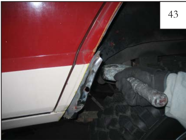
Using a hammer or mallet, pound the inner sheet metal layer over the seam.
