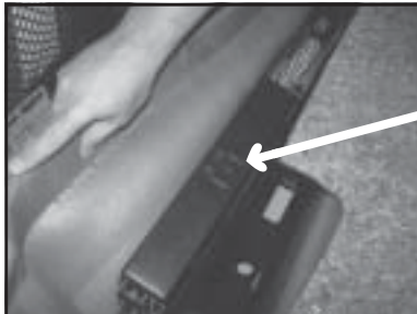
FUSE PANEL COVER PHOTO 2
