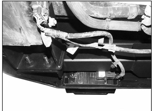
(Fig 24) Driver/left side of Bumper attached to Bumper Bracket. Sensor installation also pictured
