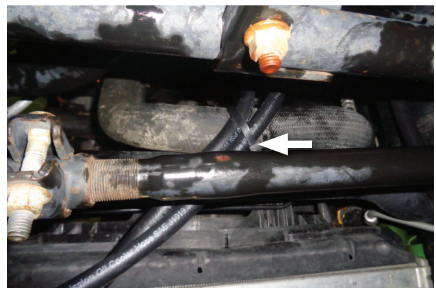
22. Correct any kinks or sharp bends in hoses then secure them with 12" cable ties as necessary.
