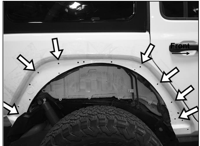
(Fig 4) Drill 25/64 hole in body panel at (7) locations (arrows). NOTE: These locations are not accessible from back of body panel
