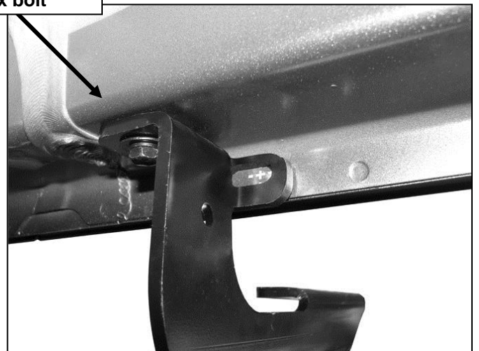
(Fig 7) Bolt the driver side center bracket in place. Mark the slot onto the pinch weld. Remove the Bracket and drill a 1/4" hole through the pinch weld
