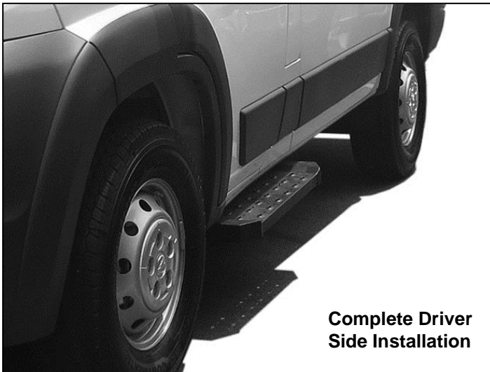
(Fig 22) Passenger side center and rear Brackets installed-mark to drill through pinch weld
