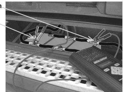
Battery Bank of 3 Batteries
