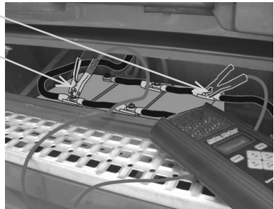
Battery Bank of 3 Batteries
