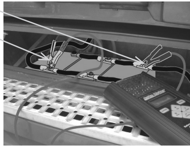
Battery Bank of 3 Batteries
