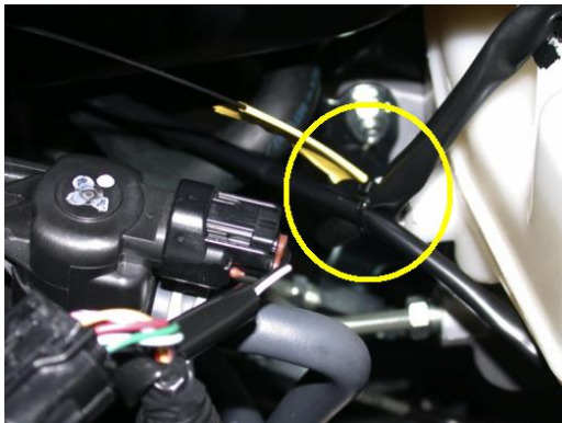
Picture 1E: wire tie left of brake reservoir
